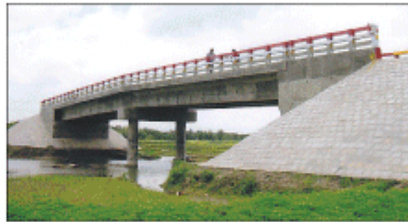
One 41.23 m long bridge on the Bhabki RHD-Raiganj GC via Beeltal Bazar Road, Melandah, Jamalpur
